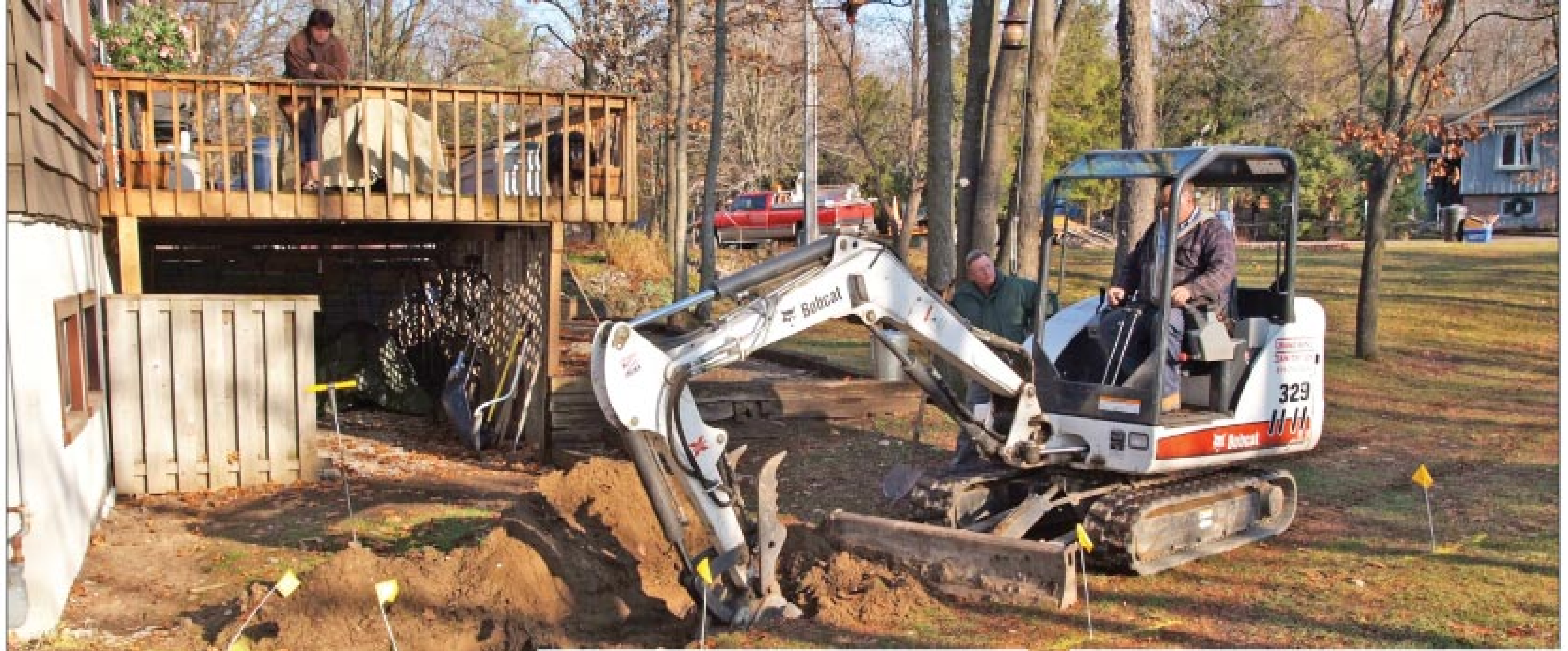
Andy O'Brien excavates a distribution box on a failing septic system. Right: Jamie Ferreira pumps a tank and cleans the distribution box while O'Brien and the homeowner look on.
