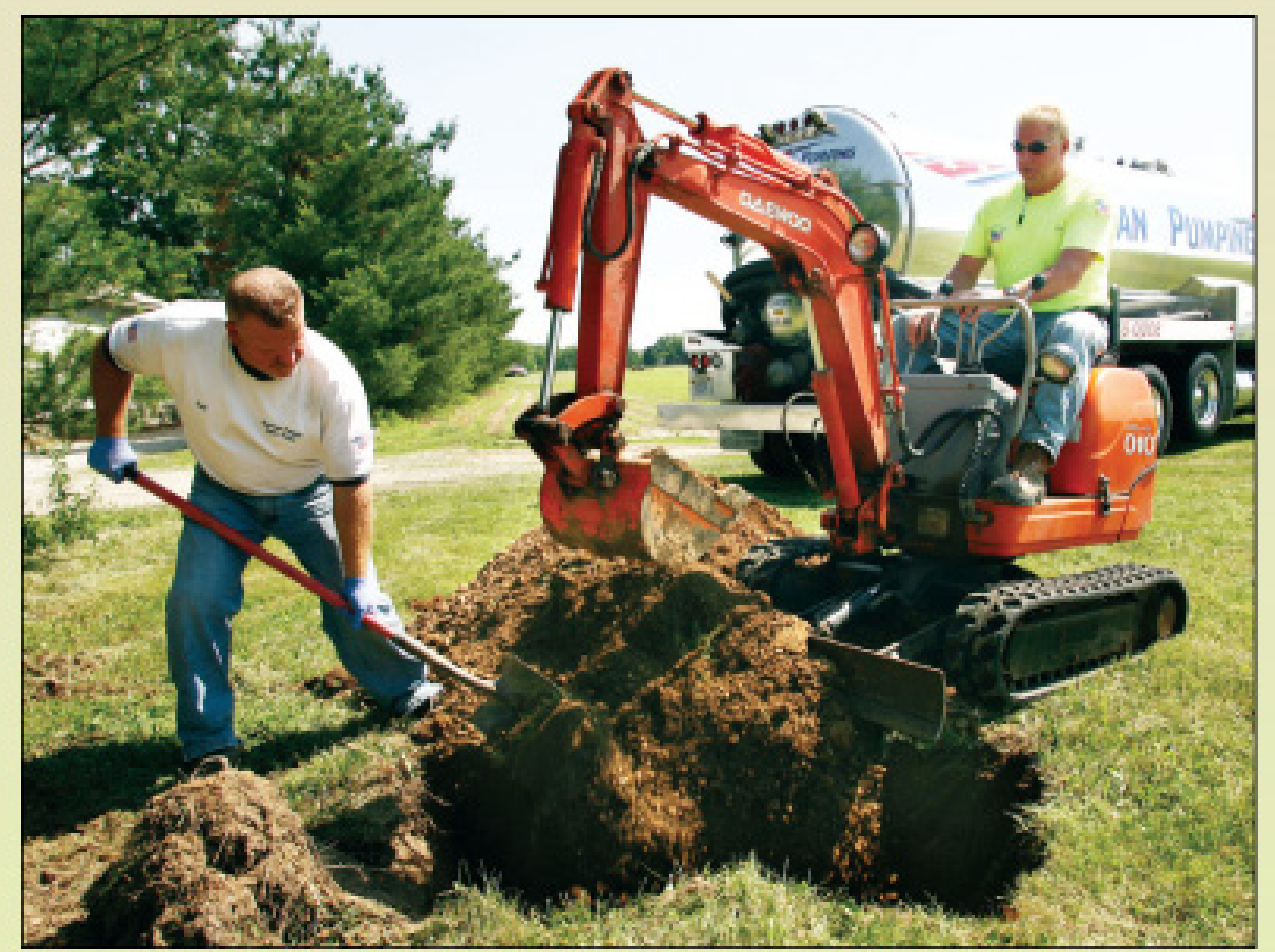
David Crume (left) and Jim Hodge backfill a tank with a Daewoo mini excavator that is transported to the site on a carrier attached to the nose of the vacuum truck.
