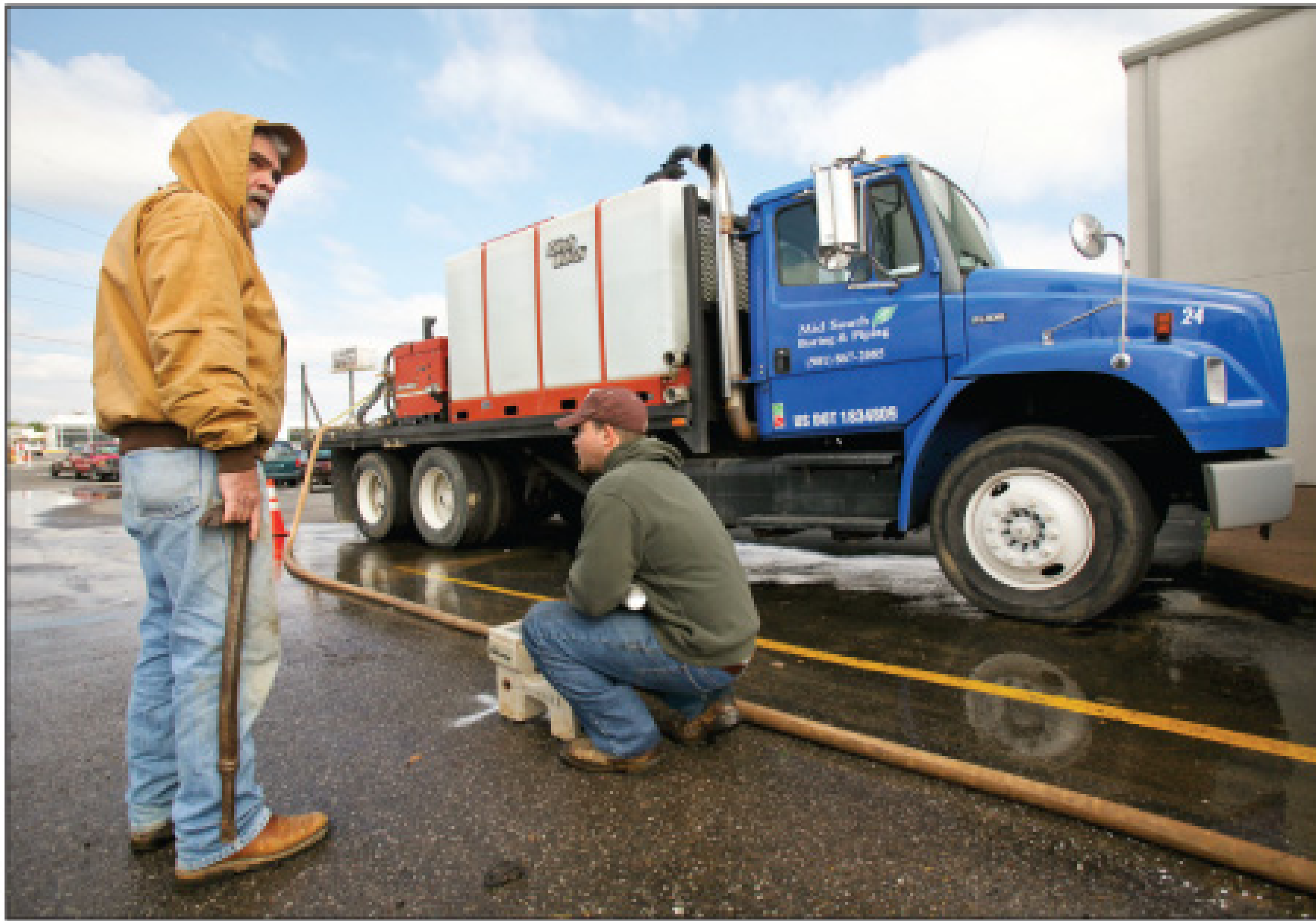
Cody Street (right) and Larry Burnette locate a pipeline under a parking lot.
