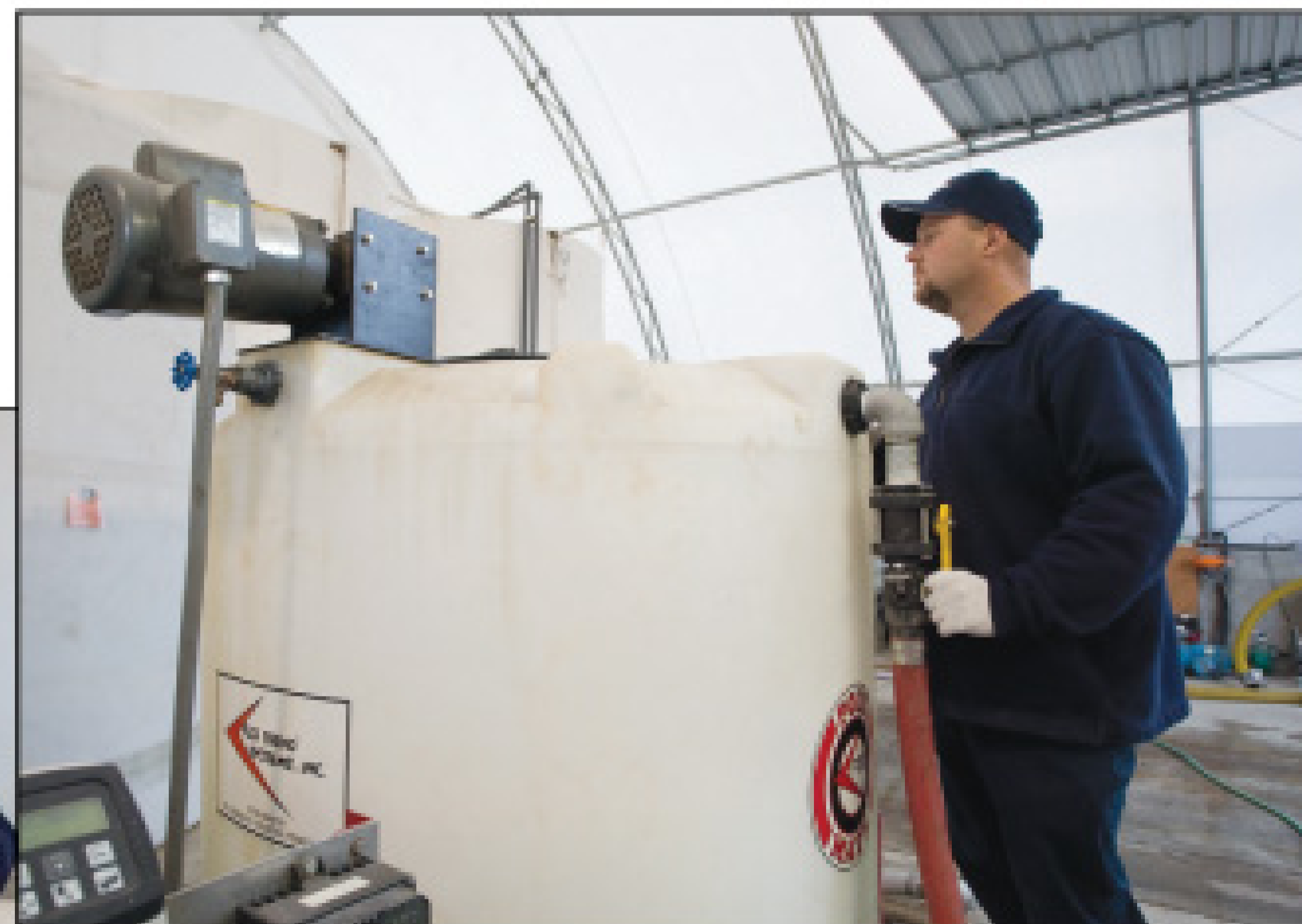
At left, Freand adds concentrated polymer to the dewatering system at the Clearwater Tech processing plant. Above, he monitors the dewatering process.
