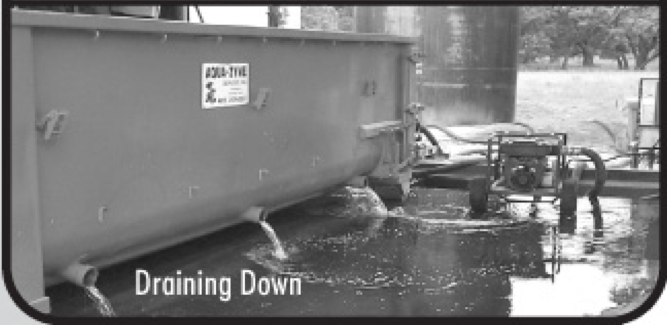
Filter Box Interior
