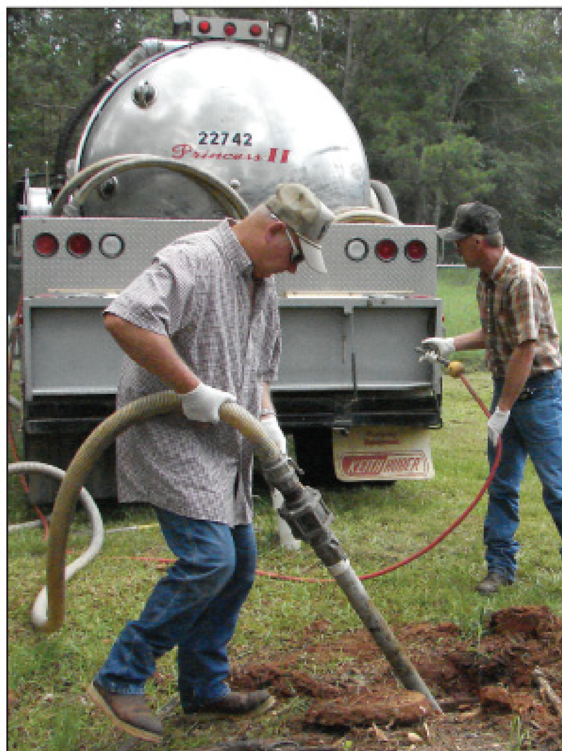
Dickerson (far left) works on a grease trap in Jasper, Texas. At left, Ward and Dickerson pump a residential septic system.
