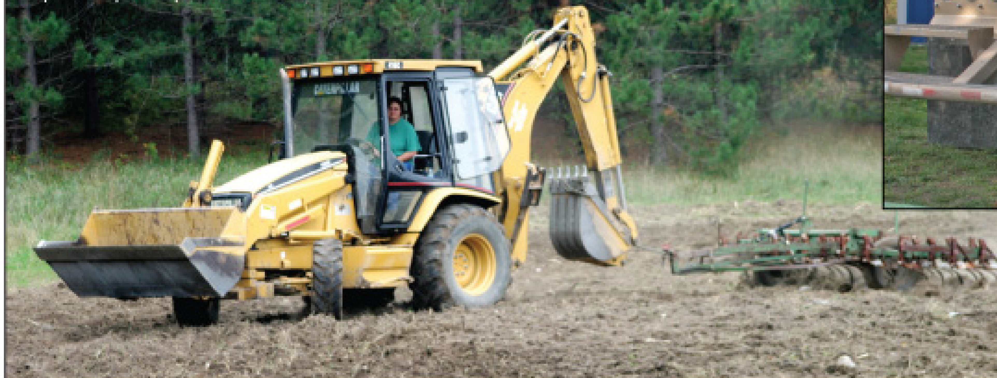
Lynn Gillespie uses a Caterpillar loader at one of two Alpena Septic disposal sites.
